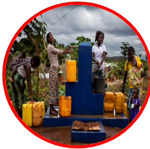
Through the construction of standpipes and household connections, residents of Bairro 4, are benefiting from an improved water supply.
