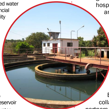
Renovating a dilapidated water treatment system provides clean water for 25,000 residents of Chimoio.
